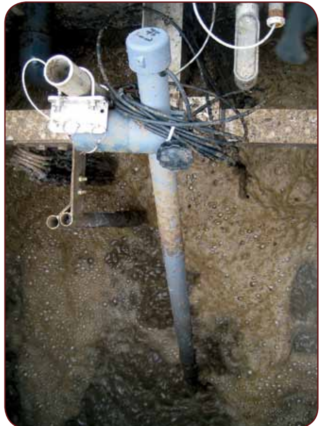
Figure 3: To prevent problems with solids content in the MBR tanks rising to excessive levels, the plant installed Hach SOLITAX sc sensors in each tank to provide continuous, real-time MLSS measurements.
