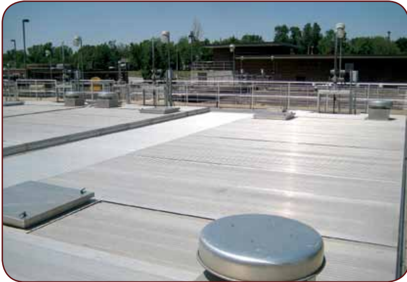
Figure 2: The plant's four MBR tanks are covered. The solids removal efficiency of the membranes allow the sludge to be contained in the system at mixed liquor suspended solids concentrations up to five times higher than possible in conventional activated sludge plants.
