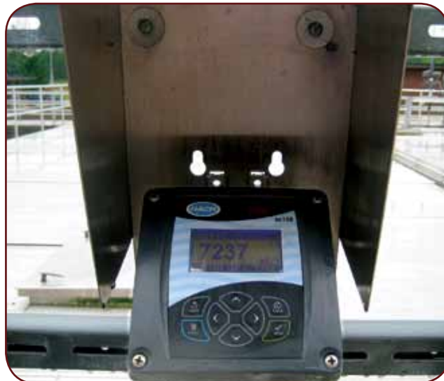
Figure 4: Hach sc100 controllers continually read the on-line SOLITAX probes and communicate this data via 4-20mA signals to the plant’s SCADA system. The controllers also have built-in dataloggers along with calibration and verification points, alarm history, and instrument setup changes for up to six months.
